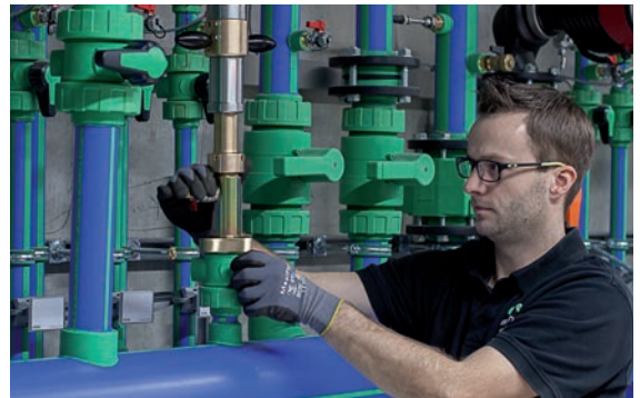
2. After the welding process and the cooling time of the weld the tapping tool is mounted on the component unit.
